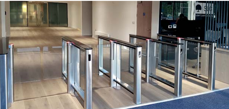
Speed gates ST-01, Office of Student Loans Company, Scotland
